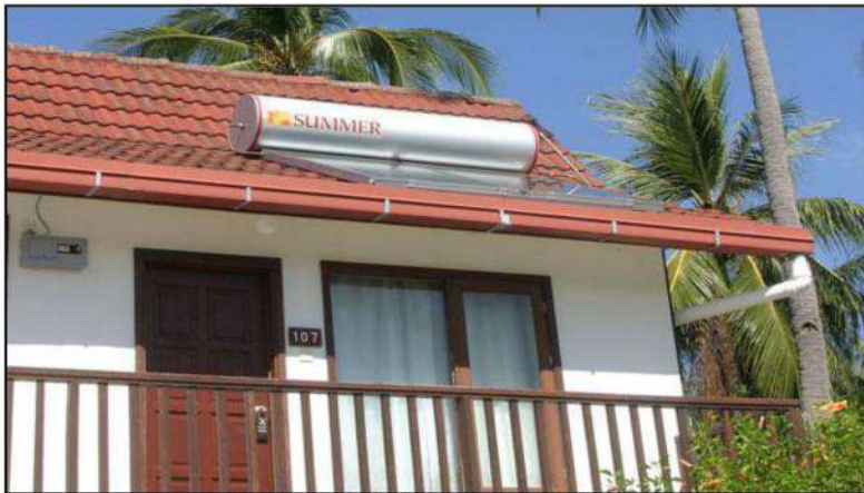
FIGURE 2 – SOLAR PANELS AT FRANGIPANI RESORT
